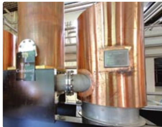
Figure 3 TVR wash condensers and flash vessels.
